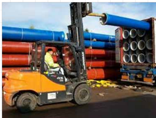
Fig. 5.2.4: Fork lift with padded booms used for unloading of pipes from trucks.
